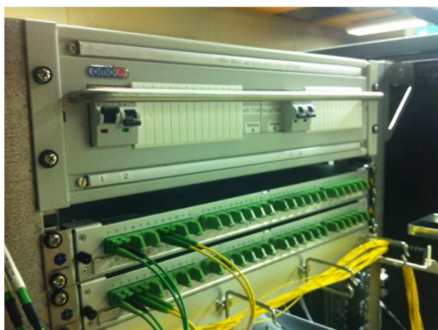
Abbildung 66 Backbone Patch Panel, CO BRE
